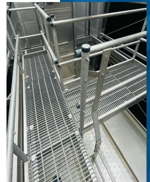
Easy and safe access via the walkway, ladder and platform
