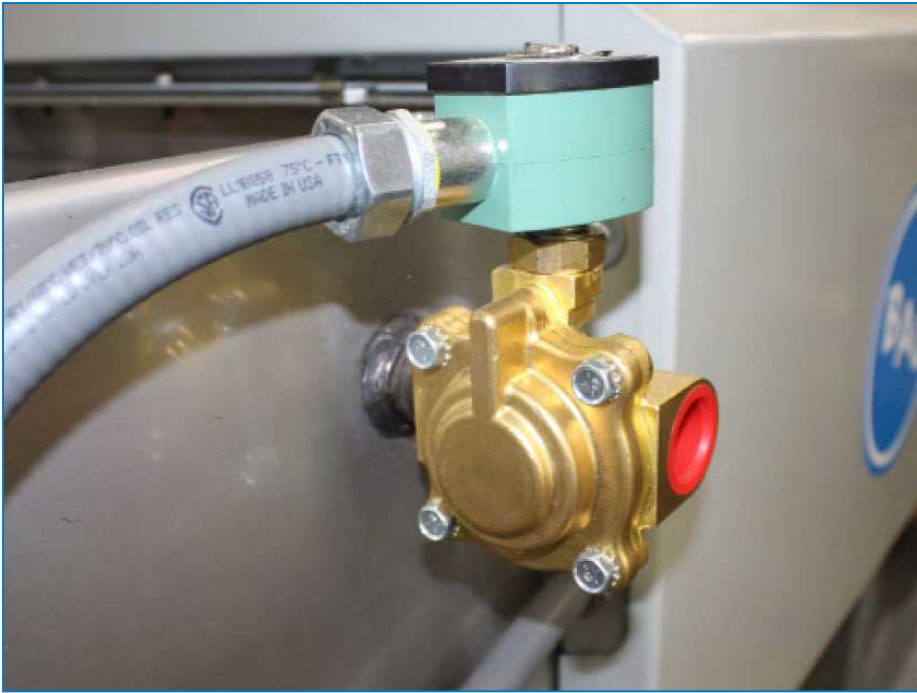
Drain solenoid valve
