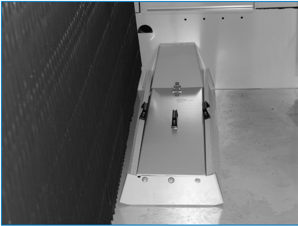
Cold water basin and basin strainer
